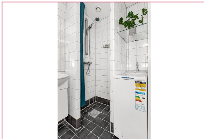
Opplegg for vaskemaskin
