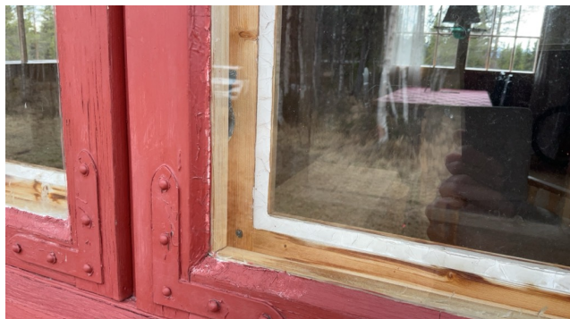
Sprekkdannelse i kitt
