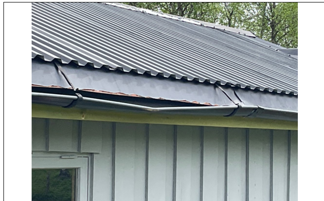
Uthus - deformerte takrenner
