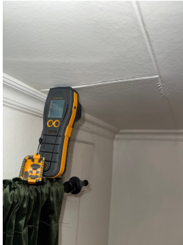
Gammel fuktskade i spisestuehimling.
