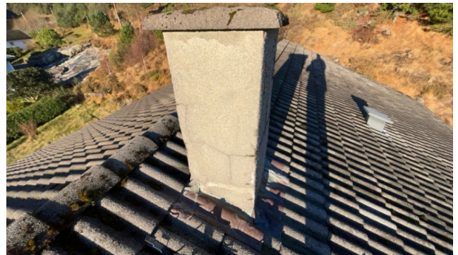
Sprekker i pipe over tak
