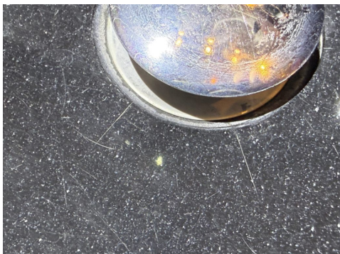
Riss/sprekker rundt servantens sluk
