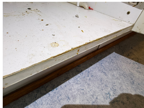
Svellinger i bunnplate under servant
