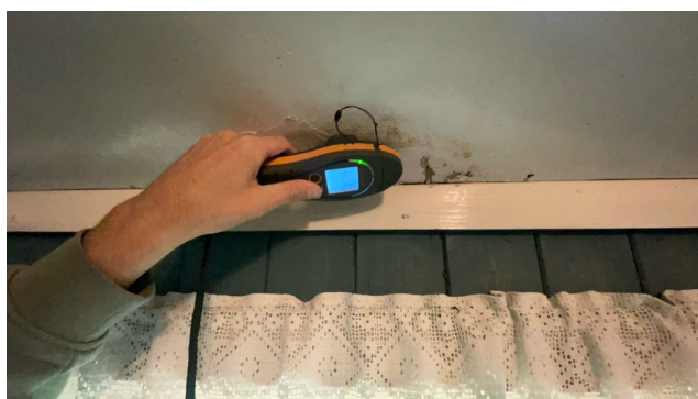
Gammel fuktskade overgang vegg/himling trapperom
