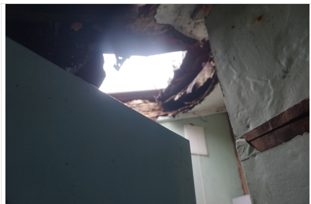
Hull i yttertaket
