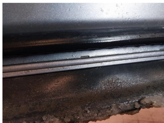
1.2 Rust i fals
