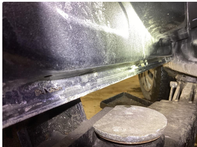
1.2 Rust i fals
