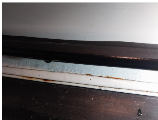
1.2 Rust i fals
