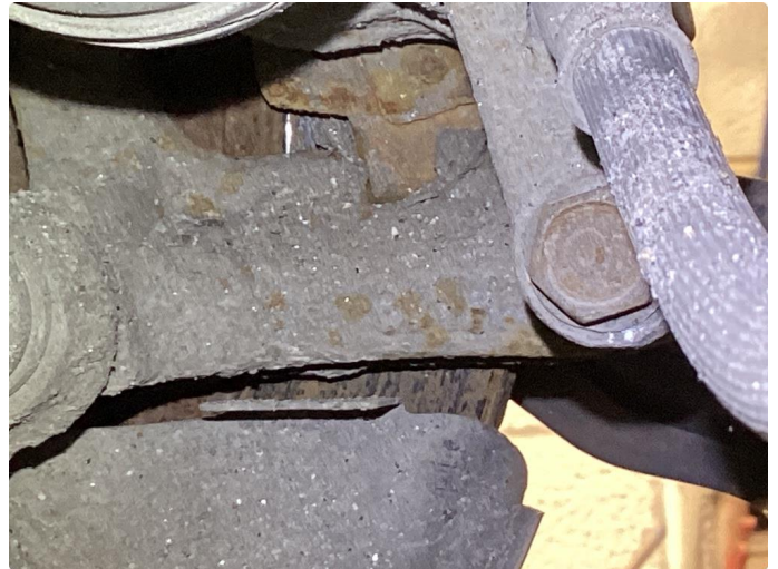
1.1 Mer enn 25% rust
