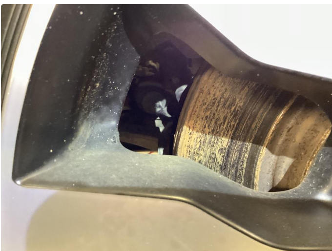
1.1 Mer enn 25% rust
