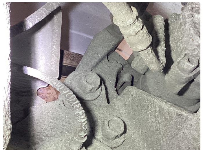
2.1 Mer enn 25% rust
