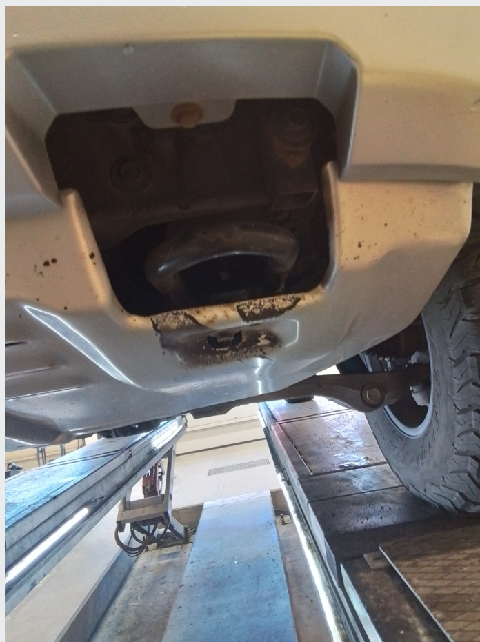
2.2 Rust bunnplate motor
