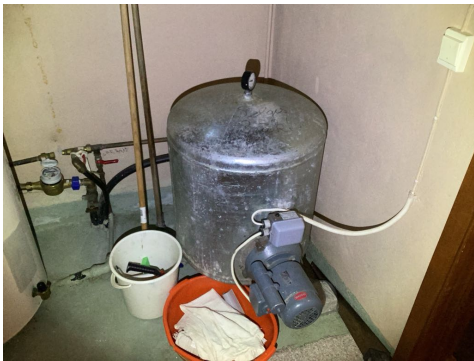
vannpumpe for brønn
