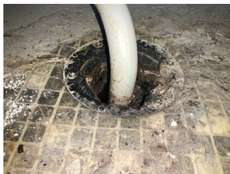
sluk under kabinett
