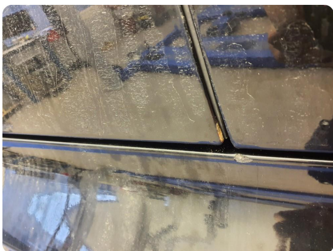
2.5 Rust i fals
