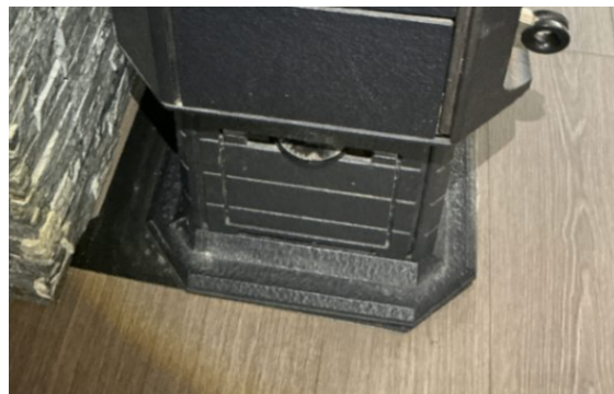
Ildfast plate feil plassert
