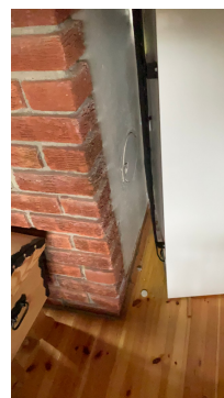
Manglende ubrennbar plate under feieluke.
