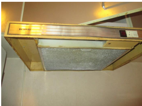
Noe eldre ventilator.
