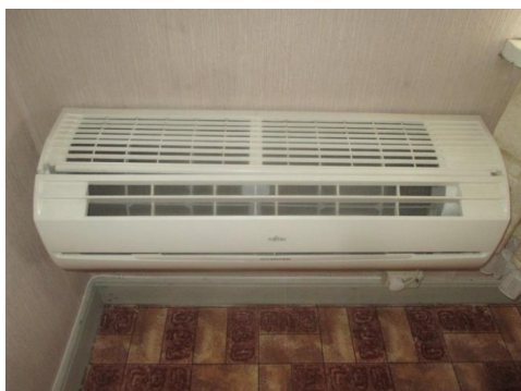
Noe eldre varmepumpe.
