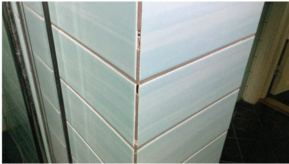
Riss i fuger.
