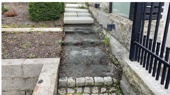
Mangler trappetrinn i steintrapp.
