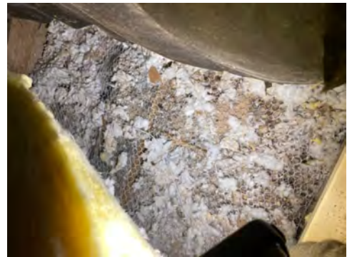
Stedvis manglende isolering.
