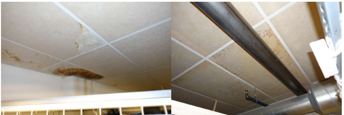
Lekkasje over systemhimling.
