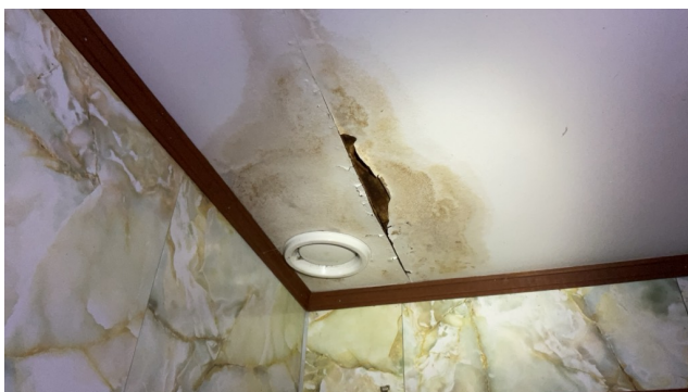
Fuktskader i himling
