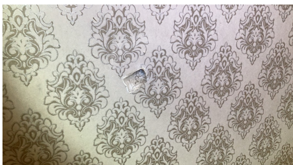
Hull i vegg.
