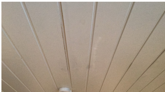
Fuktmerker i himling i stue.
