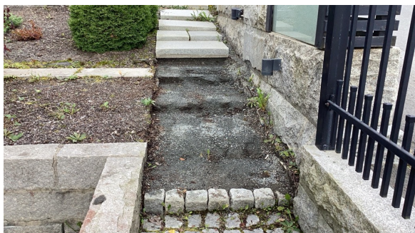
Mangler trappetrinn i steintrapp.
