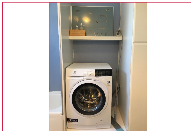
Opplegg for vaskemaskin
