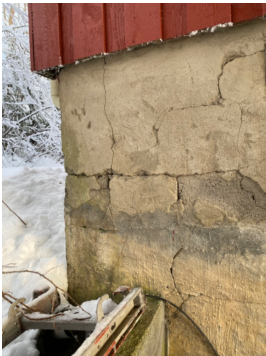
Sprekker/riss. Manglende murpuss.
