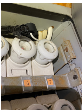
Manglende tetting rundt kabler i el.skap.
