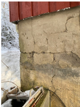
Sprekker/riss. Manglende murpuss.
