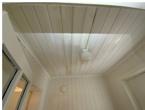
I rom under sees det fuktskjolder i panel.
