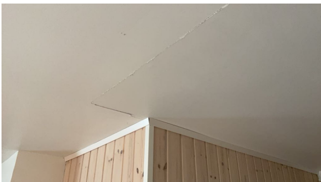
Sprekker i himling
