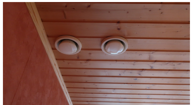
Ventiler i himling i spisesal.
