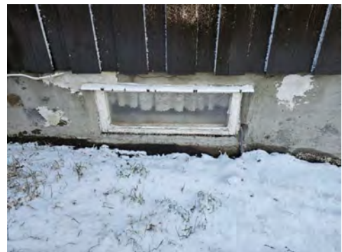
Riss/sprekk over vindu
