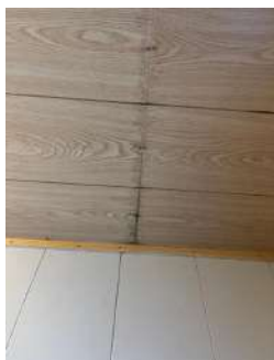
Fuktmerker i himling under balkong.
