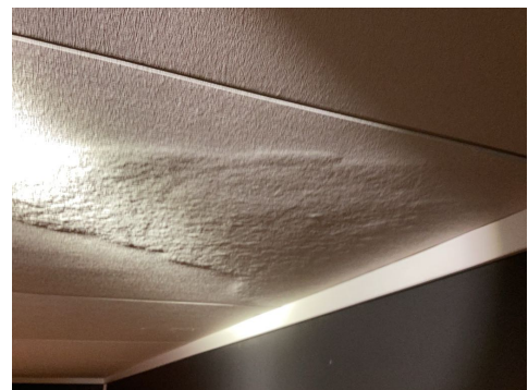
Fuktskadet himling, soverom
