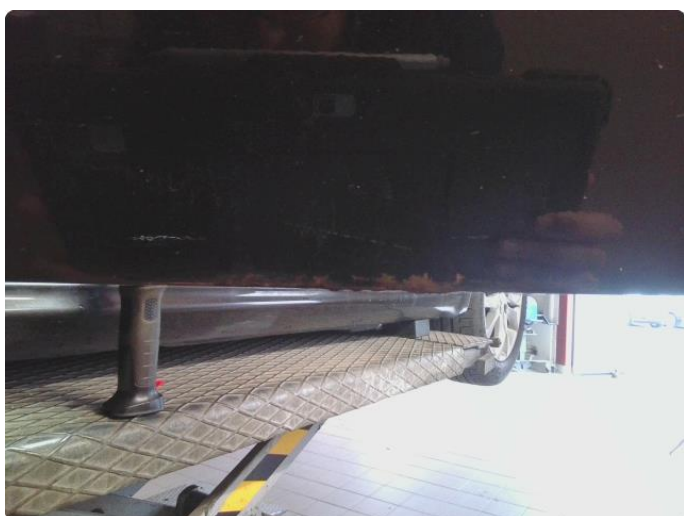
2.5 Rust i fals
