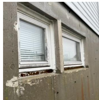
To kjellervindu mangler innpussing.
