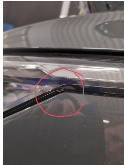
2.1 Krakelering i plast
