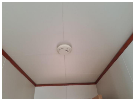
Røykvarsler montert i himling.
