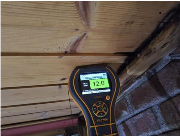
Overflater himling - [Fuktmåling, himling]
