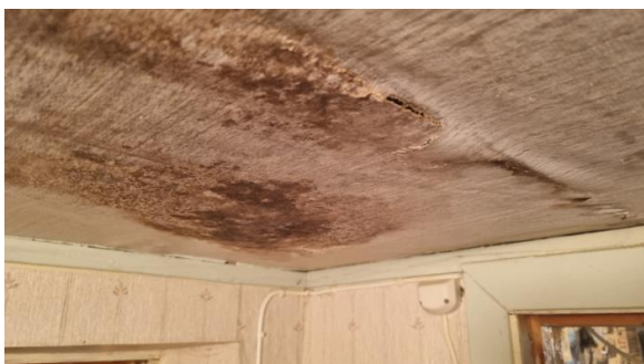
Fuktskjold/soppvekst i himling i bod under blindloft.
