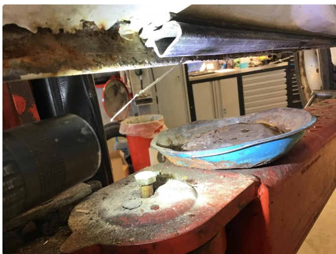
1.2 Rust i fals
