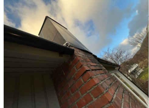
Sprekker i mur/fuger.
