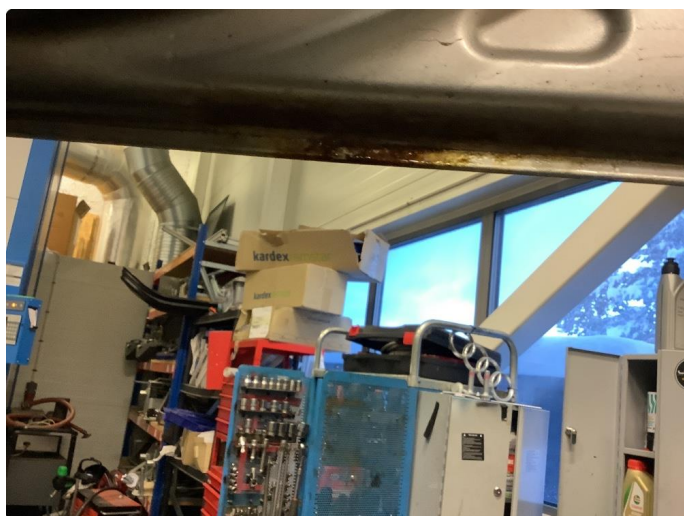
1.2 Rust i fals
