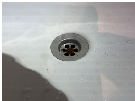
Riss/krakelering i servent.
