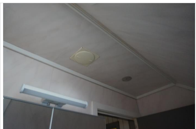
Ventil i himling.
