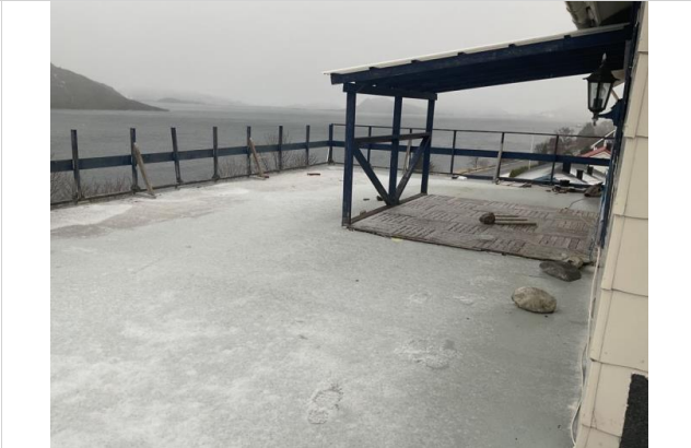
Altan, OBS mangler rekkverk
