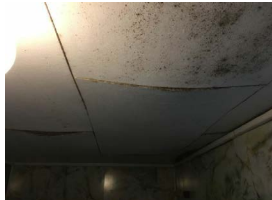
Defekte himlingsplater bad.
