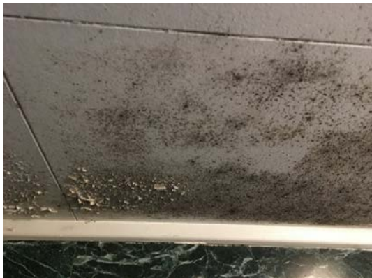
Defekte himlingsplater bad.
